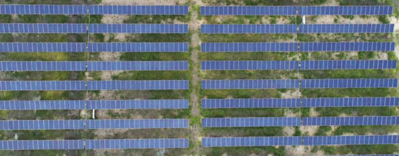
Fig. 1.22. Solar farm near Raichur, Karnataka
